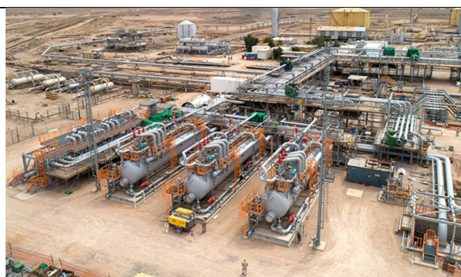
Sample of Onshore asset gas processing plant with production wells, connector and export pipelines
