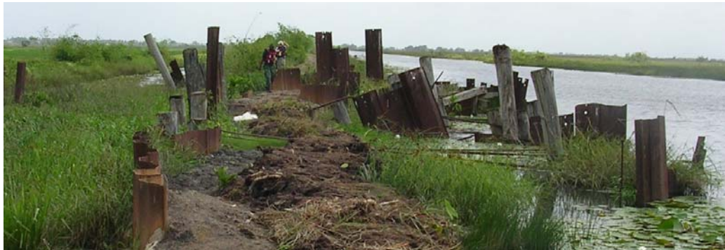
The state of the Conservancy dam is characterized by poor maintenance and patchwork and requires urgent repair
