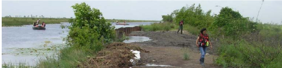
The dam, with at the conservancy swampland and at the right the coastal zone. White bags with clay and some peat are retaining the water. In the back an overtopping, sealed of with sheet piling works
