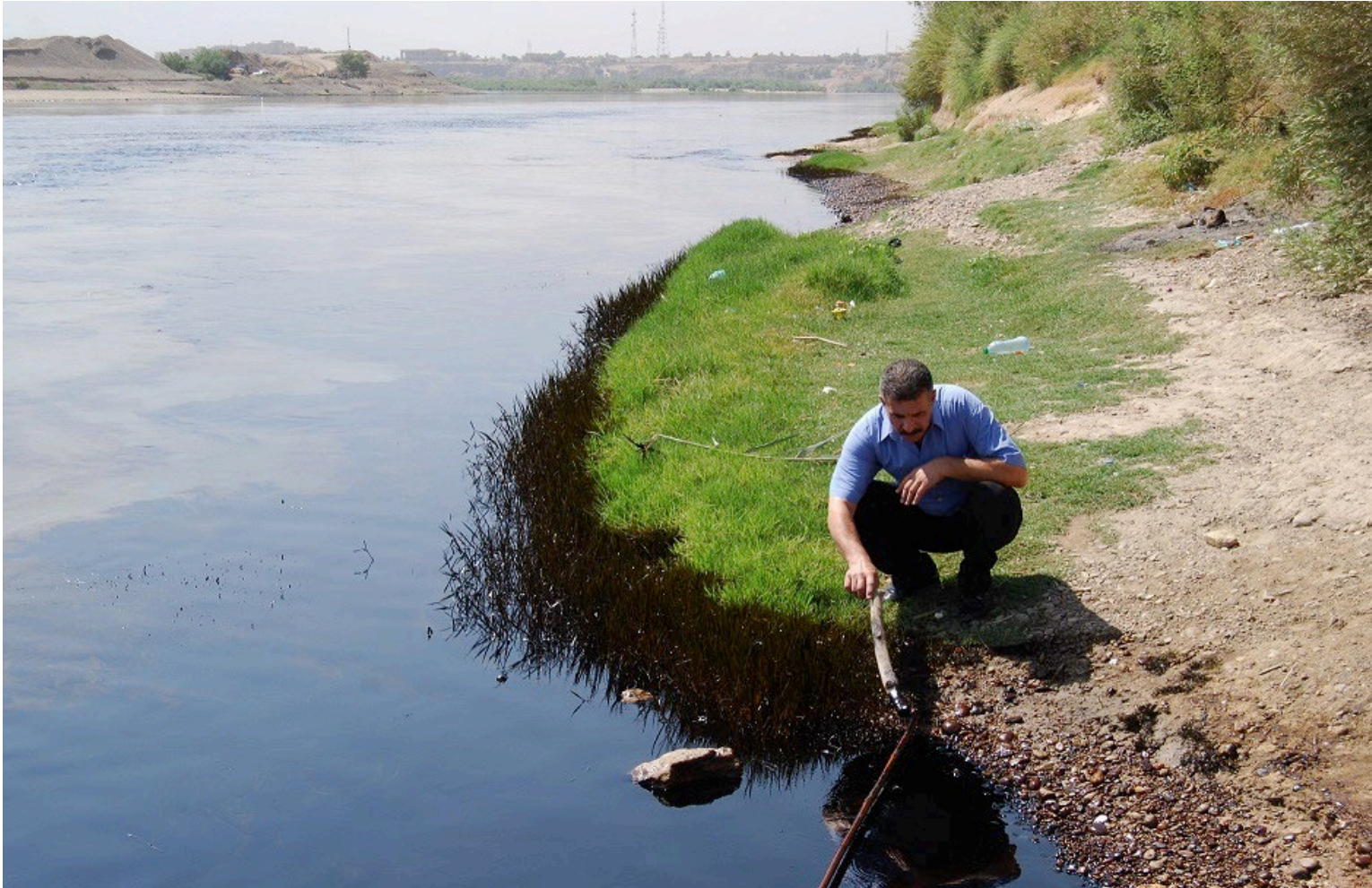
River-crossing crude oil pipeline failure causing spillage directly into river
