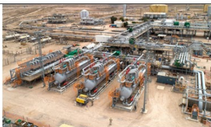
Sample of Onshore asset gas processing plant with production wells, connector and export pipelines
